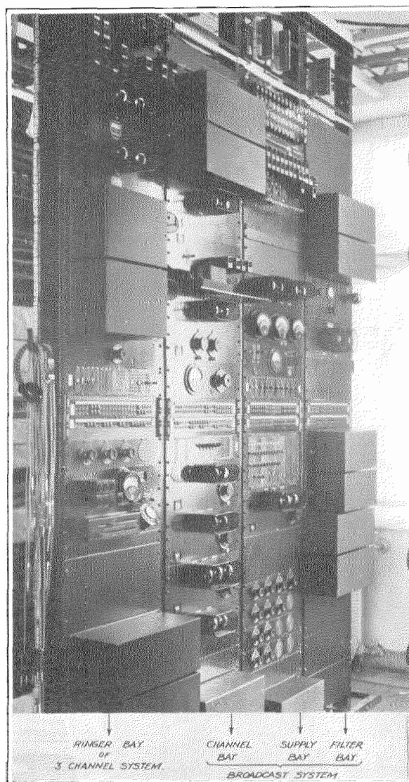
Figure 5—Carrier Broadcast Equipment at Bratislava.
